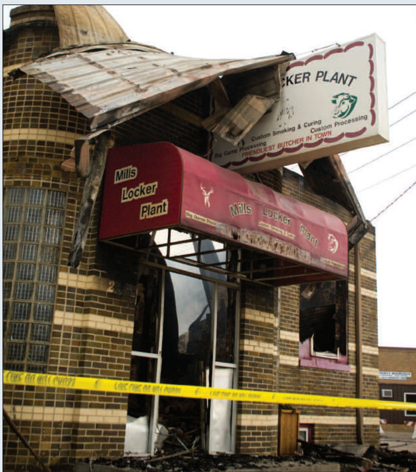
The Mills Locker Plant has been a staple in New York Mills for decades.
